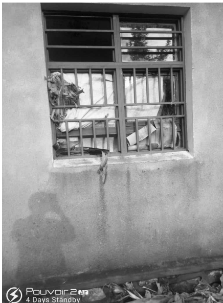
Damaged window at the ranger post
