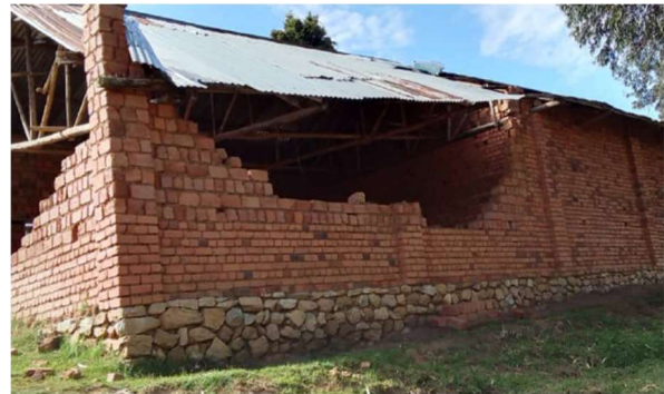
A building of the Mt. Tshiaberimu school, badly damaged by a storm © Kasereka Gervais
