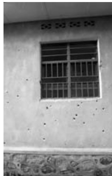
Damage that the fights caused in the Sarambwe patrol post
